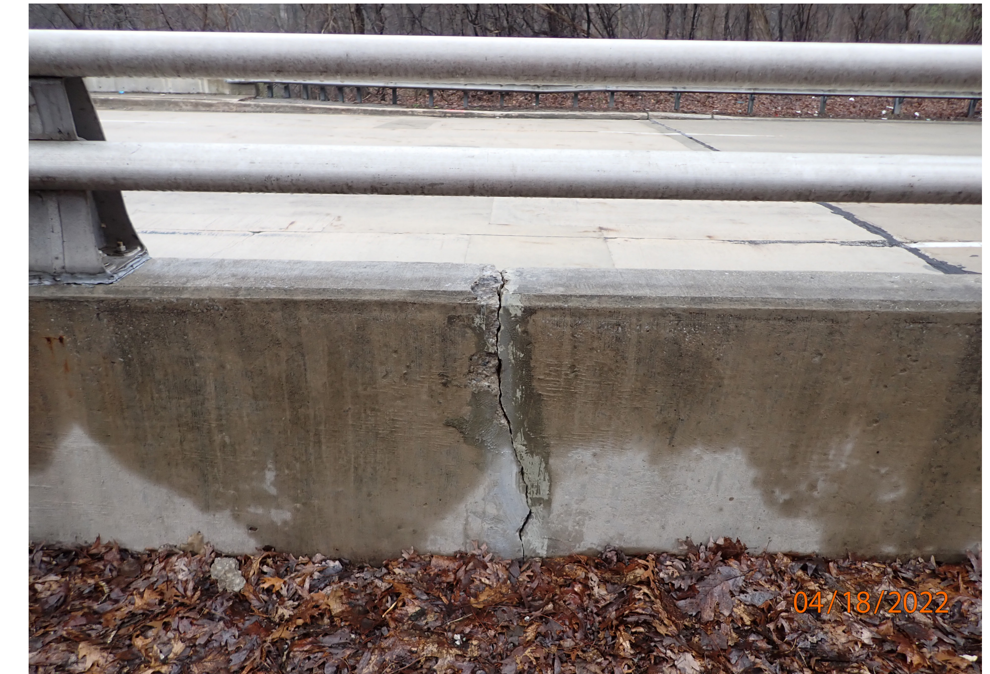
Typical vertical crack in parapets
