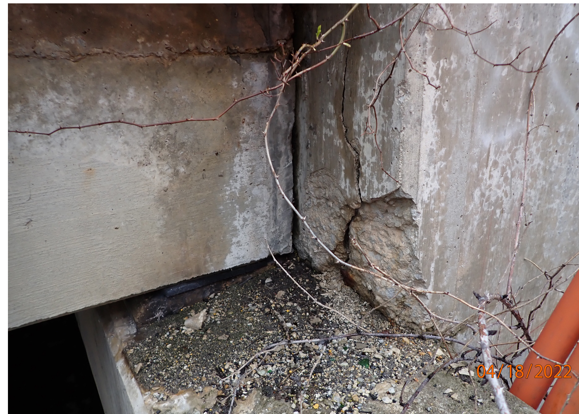
Abutment backwall spalling near Precast Prestressed Concrete
