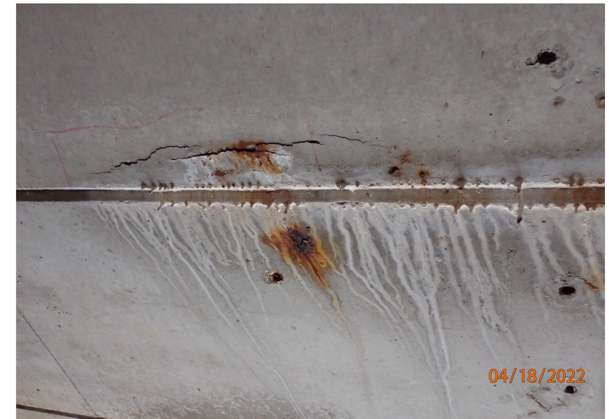
Delamination and rust staining on underside of Precast Prestressed Concrete beam
